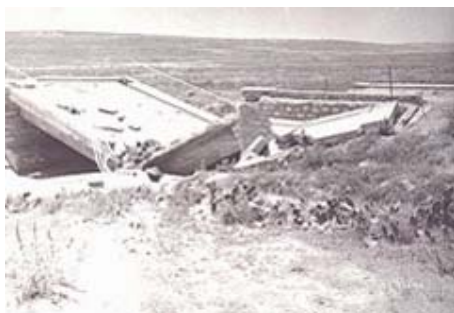
Blown bridge Sousse-Tunis Road
